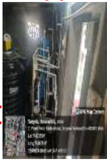
RO water plant
