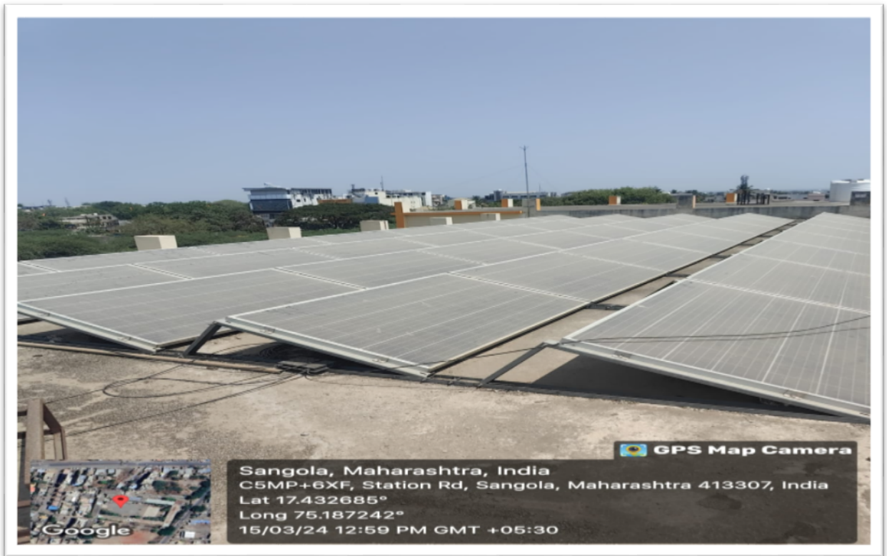
Fig.15: Solar panels on college building roof
