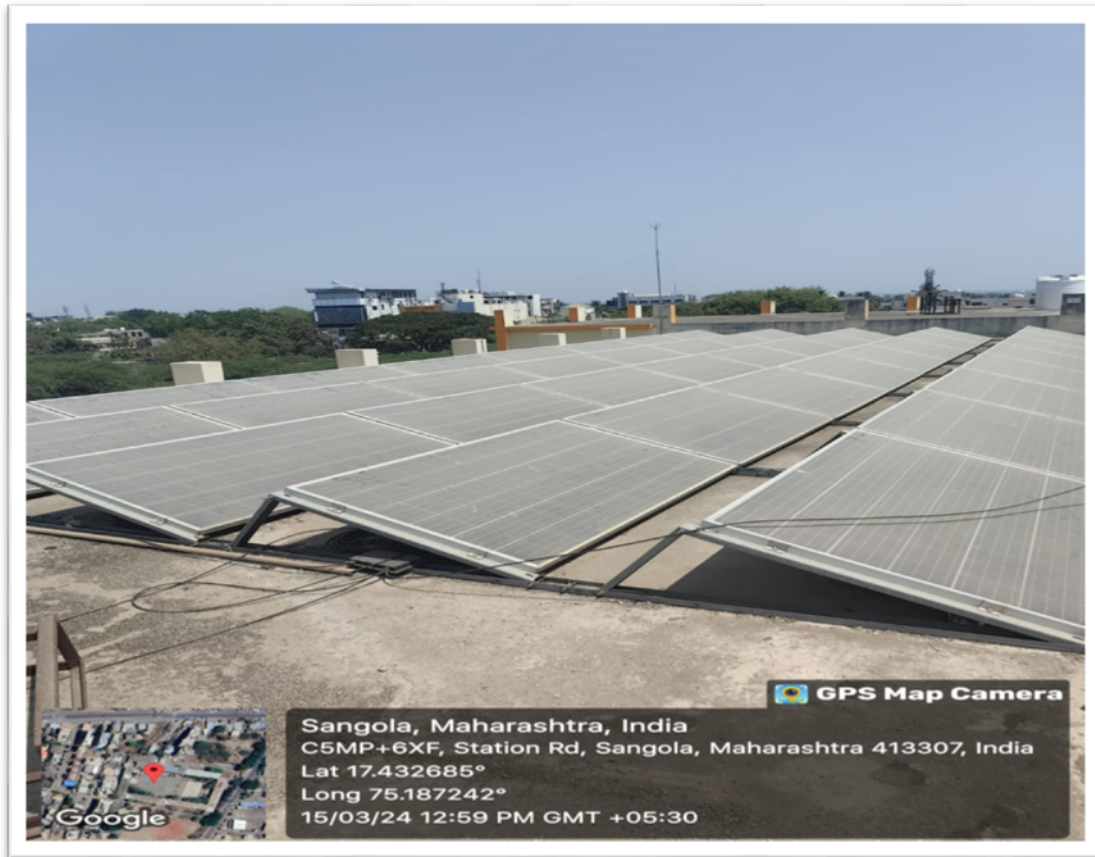
Fig. 22: Solar Panels on the College Building Roof
